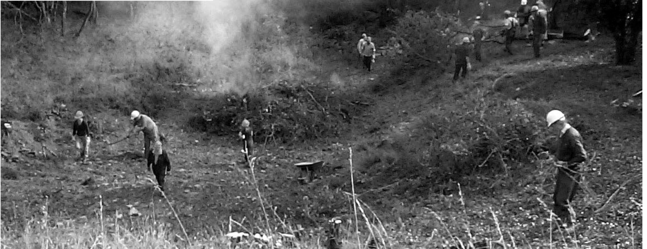
THE LOWER CANAL BASIN OF THE FUSSELLS BALANCE LOCK SITE COMES TO LIGHT — October 2003 Inset: BEFORE CLEARANCE — January 2002
