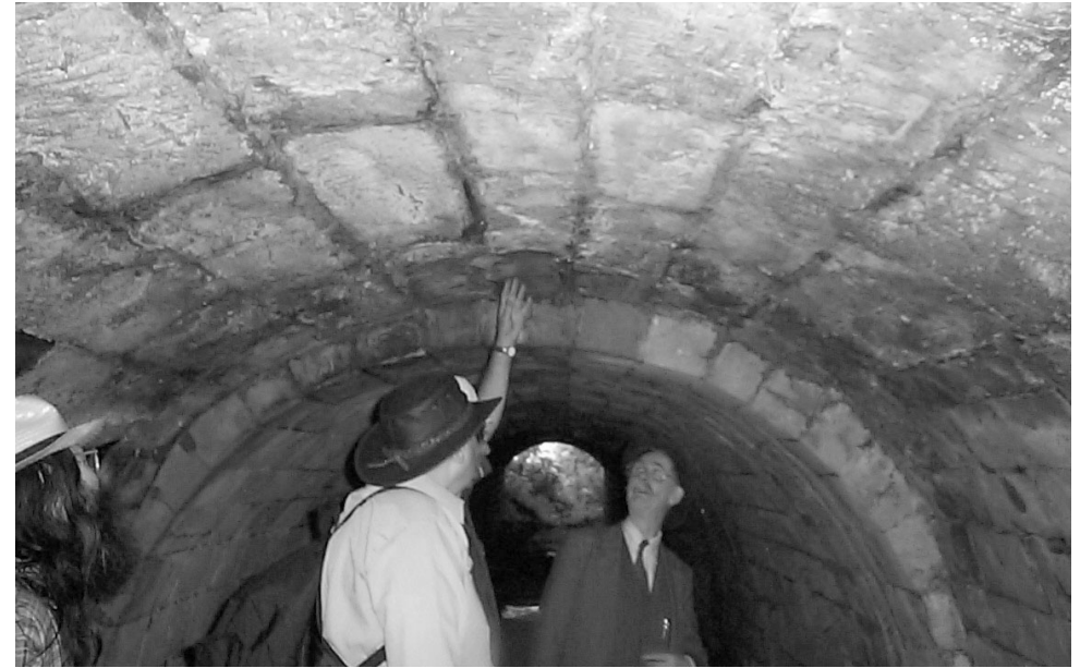
COMBE HAY AQUEDUCT TUNNEL Showing a junction of the original canal structure with a later construction, probably when the embankment was widened for the railway
