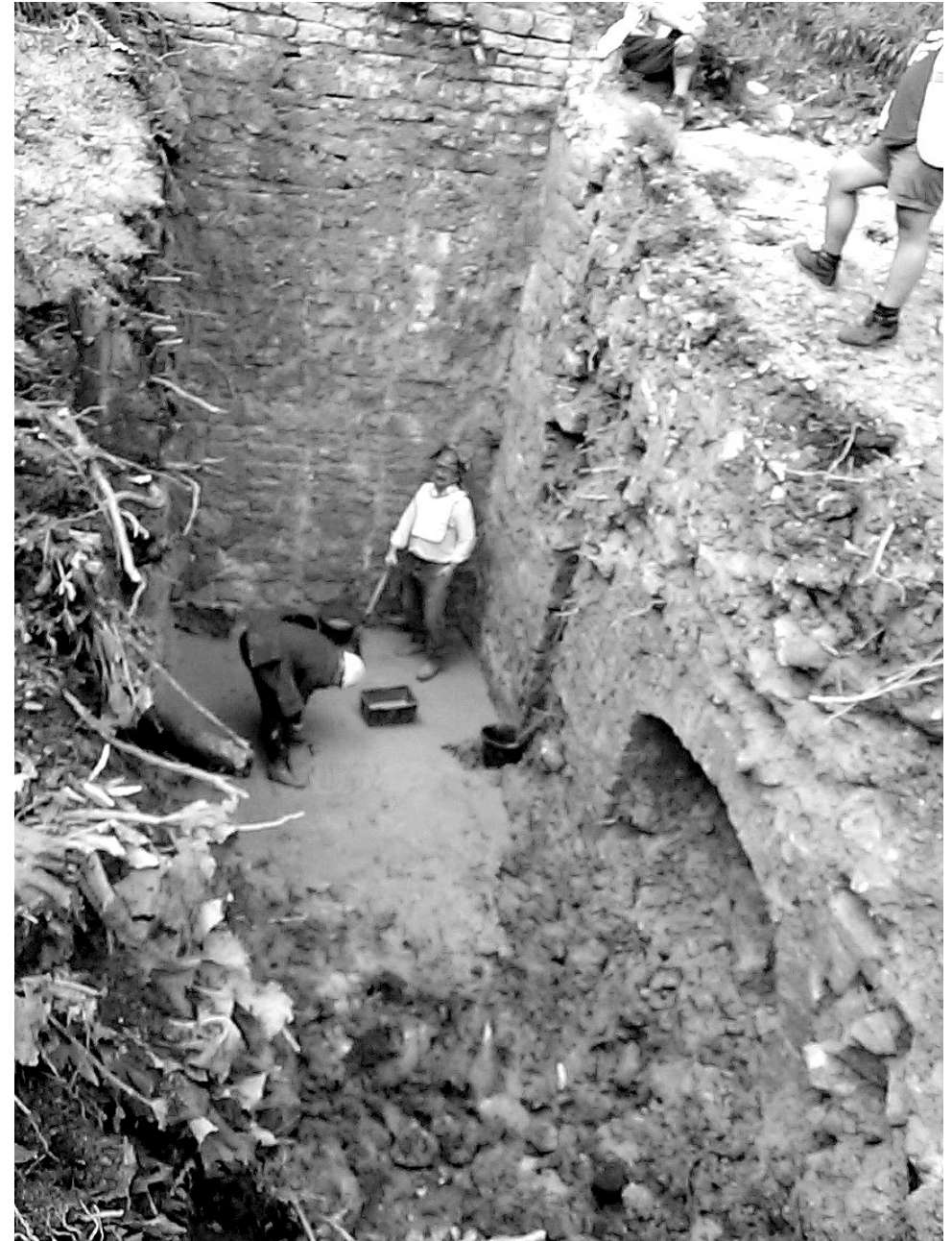
THE LOCATION OF FUSSELS TRIAL BALANCE LOCK HAS BEEN CONFIRMED BY THIS SPECTACULAR EXCAVATION ON THE DORSET & SOMERSET CANAL A full report follows in the next issue.
