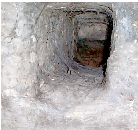
THE HOLE IN THE CANAL TUNNEL ROOF SEEN FROM BELOW
