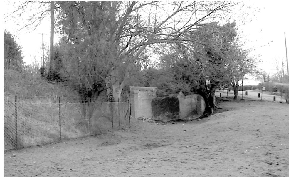
DRAMWAY TUNNEL TO AVON WHARF - under the A4175 road near Chalk Mill Farm
