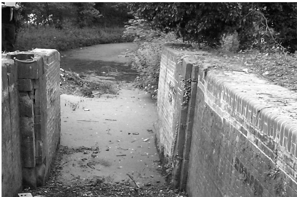
CALNE TOWN LOCK with the newly-restored canal beyond. Note the top hinge strap in place, ready to receive a new gate
