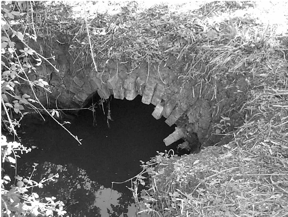
ONE END OF THE COLLAPSED CULVERT
