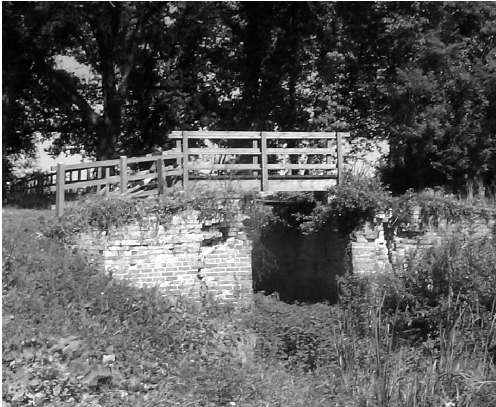
TOP LOCK OF THE PEWSHAM FLIGHT A modern bridge over the bottom end
