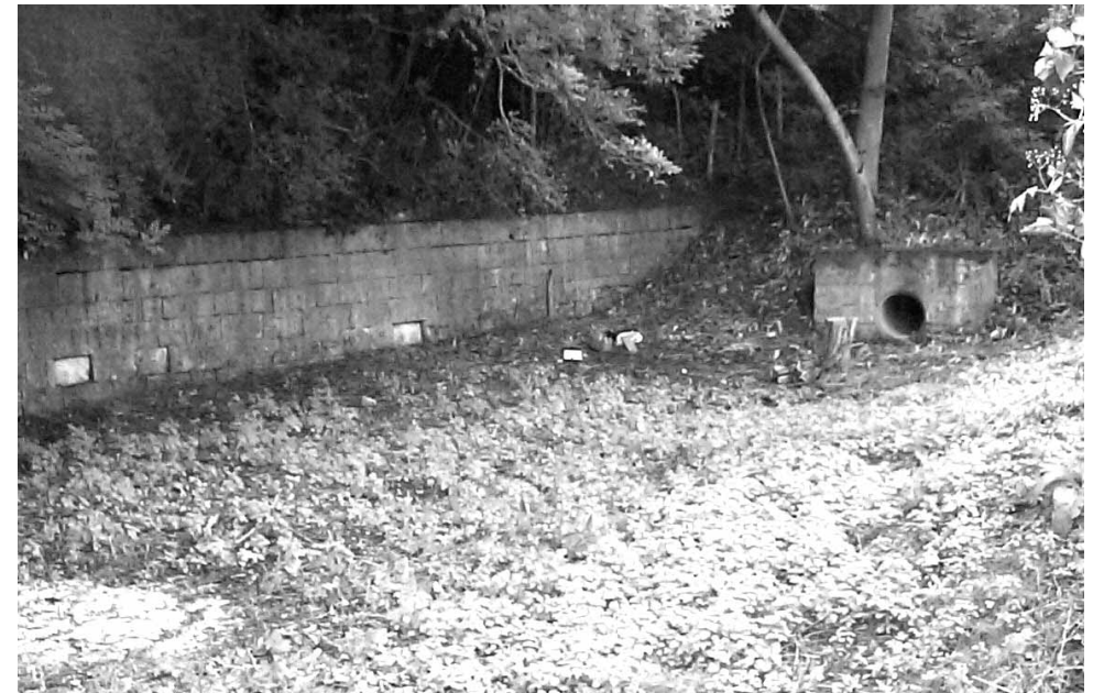
THE TOWPATH WALL BELOW LOCK 19 AND THE CONCRETE PIPE WHICH REPLACES SOUTHSTOKE BRIDGE
