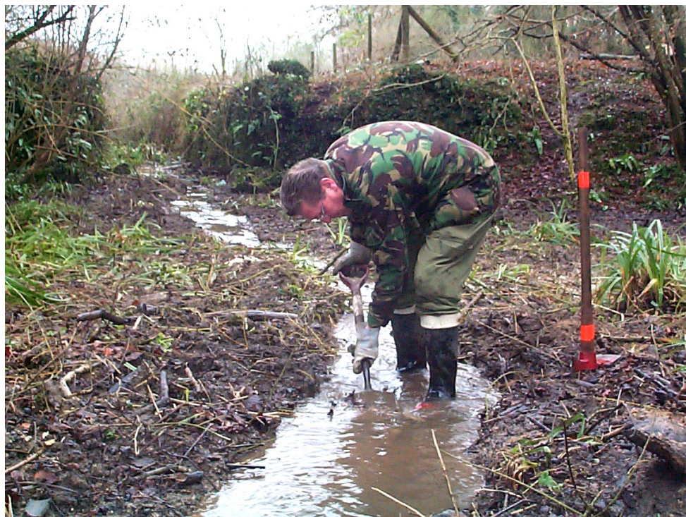
WORK AT THE BULL'S NOSE — January 2008 Bob Parnell attempting to re-open the canal single-handedly?
