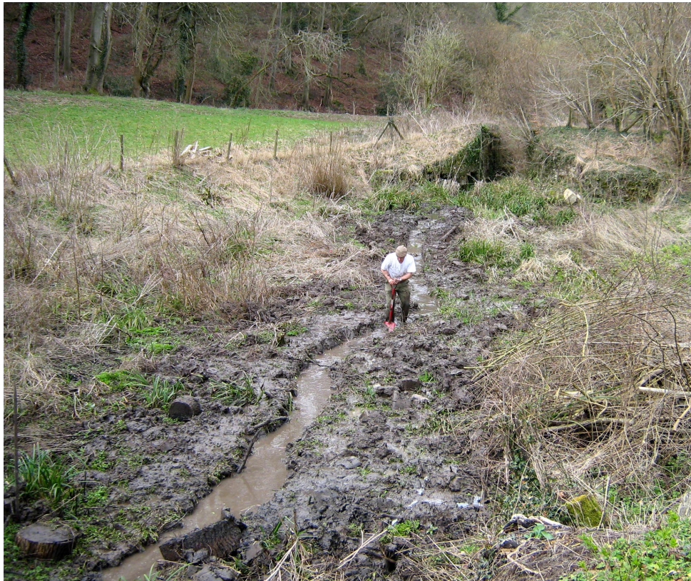
Photograph: P. Hucklebridge A SEA OF MUD — Richard Hignett digging a channel across the pound between Lock 11 and Lock 12
