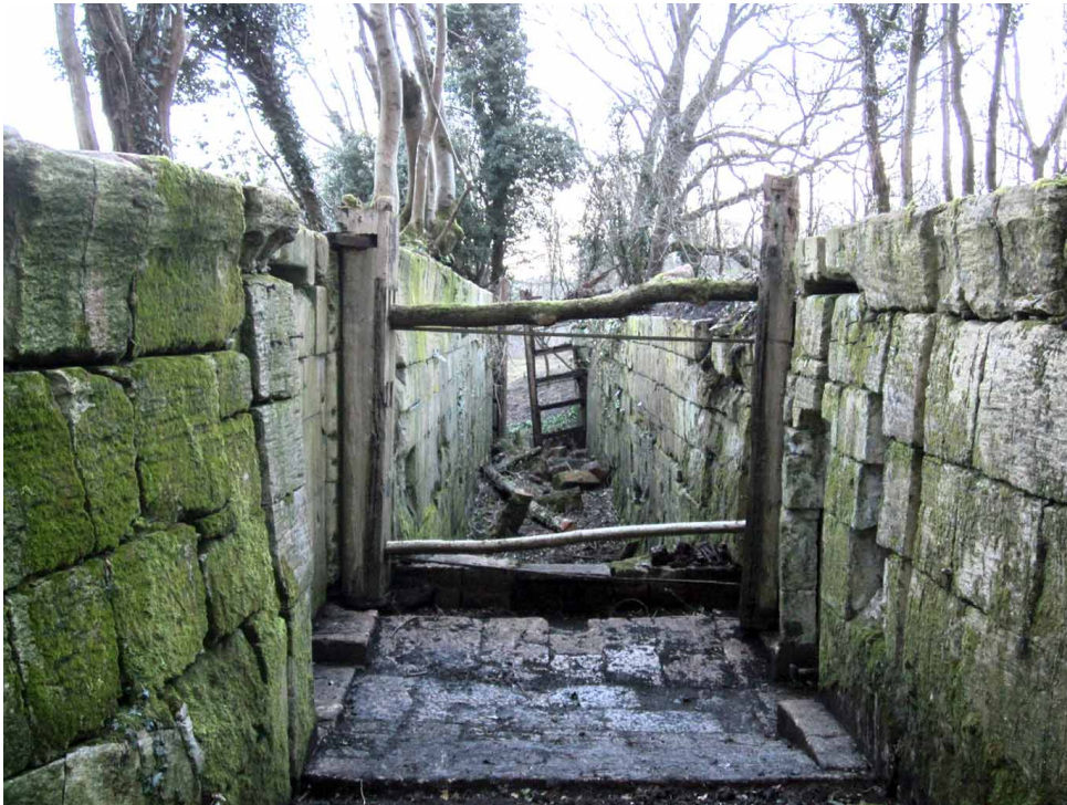
LOCK 2 RECENTLY UNCOVERED Showing the remains of the bottom and top gates still in place
