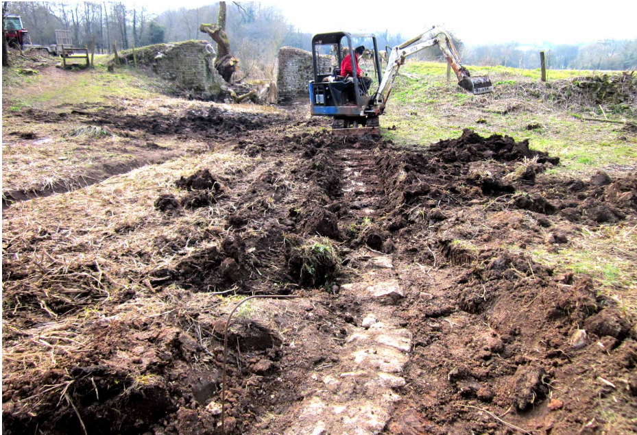
View 1 — THE NORTH WALL OF THE DRY DOCK EXPOSED DURING EXCAVATIONS The inner face [left side in this picture] was found to be much rougher than the outer face, probably having been robbed of its good quality facing stone
