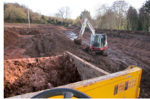
A VIEW OF THE DIGGER FROM THE SEAT OF THE DUMPER — The digger is lifting spoil up the embankment and the topsoil is piled to the left of the picture
