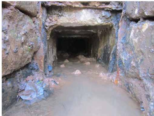
A VIEW DOWN THE DRAIN NEAR TERMINUS BRIDGE With rotted ironwork and displaced and leaking masonry
