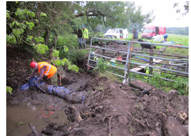
A BIG MUDDY HOLE WHERE THE TREE STUMP HAD BEEN. W.R.G.IES PREPARING TO BUILD A DAM TO KEEP THE STREAM OUT OF THE WORK AREA.
