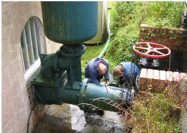
WORK IN PROGRESS ON THE CLAVERTON PUMP SHOWING THE IMMENSE SIZE OF THE FITTINGS
