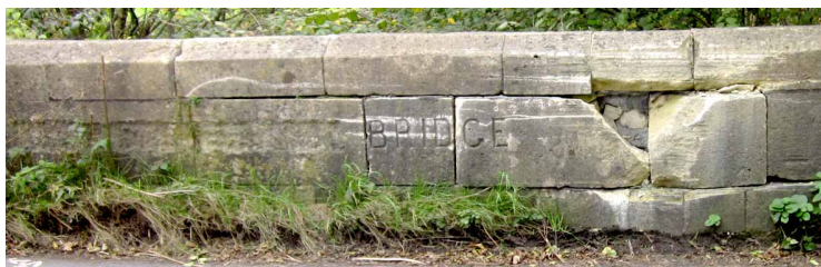
[Right] THE DEFACTED CARVING ON THE BRIDGE PARAPET
