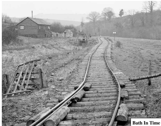
Fig. 8 — UNEVEN TEMPORARY TRACK NEAR LOCK 22
