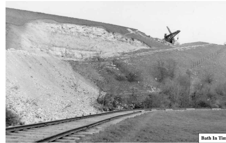
Fig. 9 — A STEAM NAVVY DIGGING INTO THE HILLSIDE ABOVE UPPER MIDFORD, EAST OF LOCK 22 THE TEMPORARY RAILWAY IS IN THE FOREGROUND
