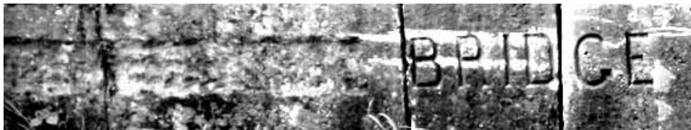
THE DEFACED NAME CARVED ON THE PARAPET OF COMBE BRIDGE
