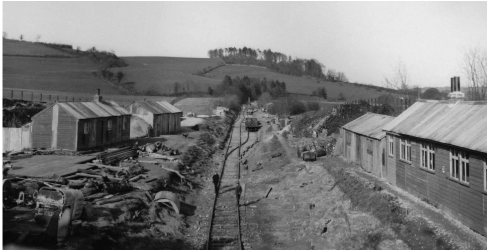
Fig 26 — VIEW OF THE CONTRACTOR'S DÉPÔT LOOKING EASTWARDS FROM THE PARAPET OF COMBE HAY TUNNEL
