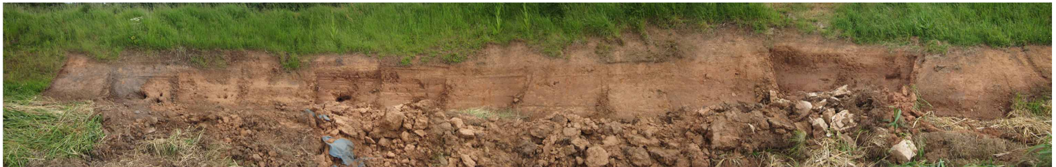
A PANORAMIC VIEW OF THE LEAKING SECTION OF CANAL BANK AT WITHY MILLS
