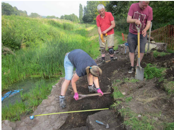
S.C.C.S. VOLUNTEERS DOING THE BACK-BREAKING WORK OF EXCAVATING THE TOP OF THE ABUTMENTS OF TERMINUS BRIDGE
