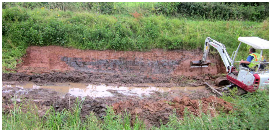
Fig 4 — CANAL EMBANKMENT SHOWING PATTERN OF COAL WASTE INFILL
