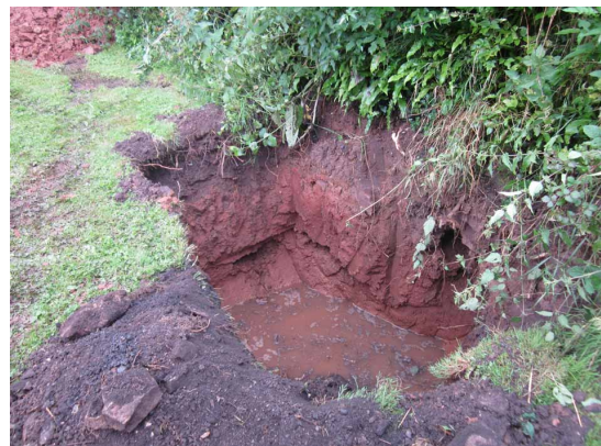
Fig 5 — THE LEAKS COMBINING IN PASSAGeways ON THE DOWNHILL SIDE OF THE CANAL EMBANKMENT
